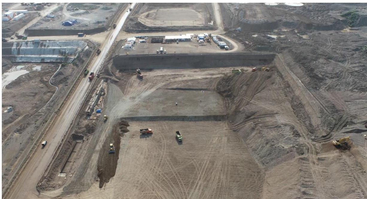
Figure 2: Aerial View of the AIM Acid Plant Earthworks and Retaining Walls Underway
