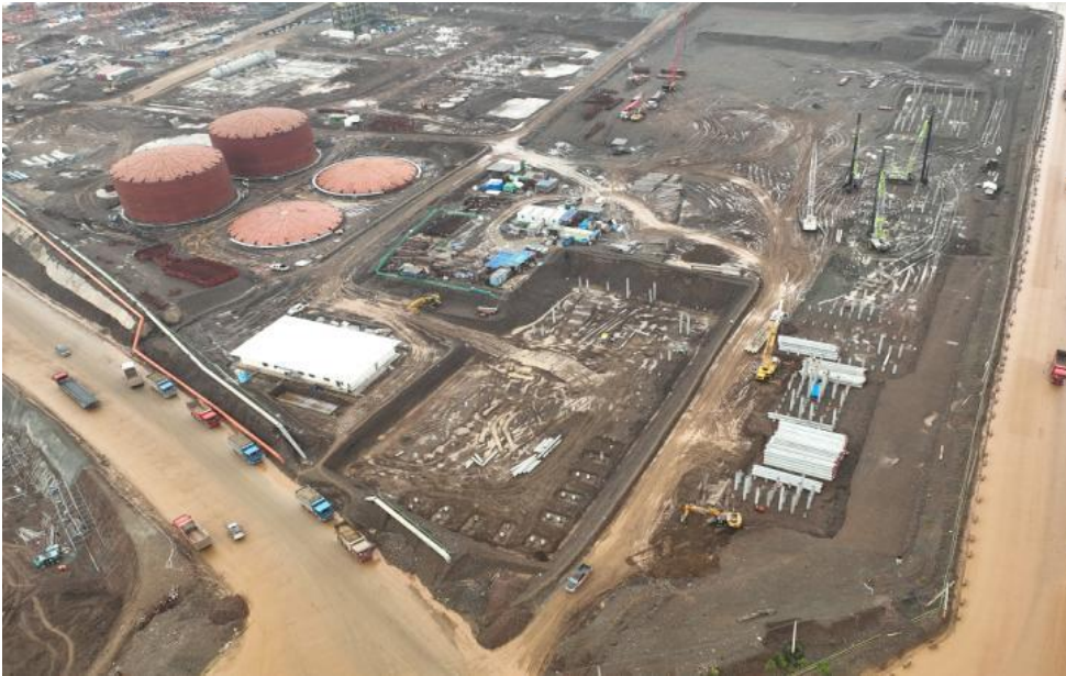
AIM Acid Tanks and Chloride Plant
