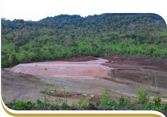
Heap Leach Pad - all works completed to the extent of the IPPKH 194 Ha perimeter
