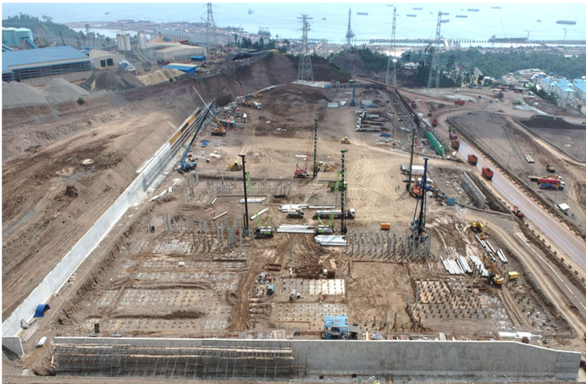
Figure 4: AIM Acid Plant: Perimeter retaining walls, piling for 2 x Acid Trains and Gas Purification
