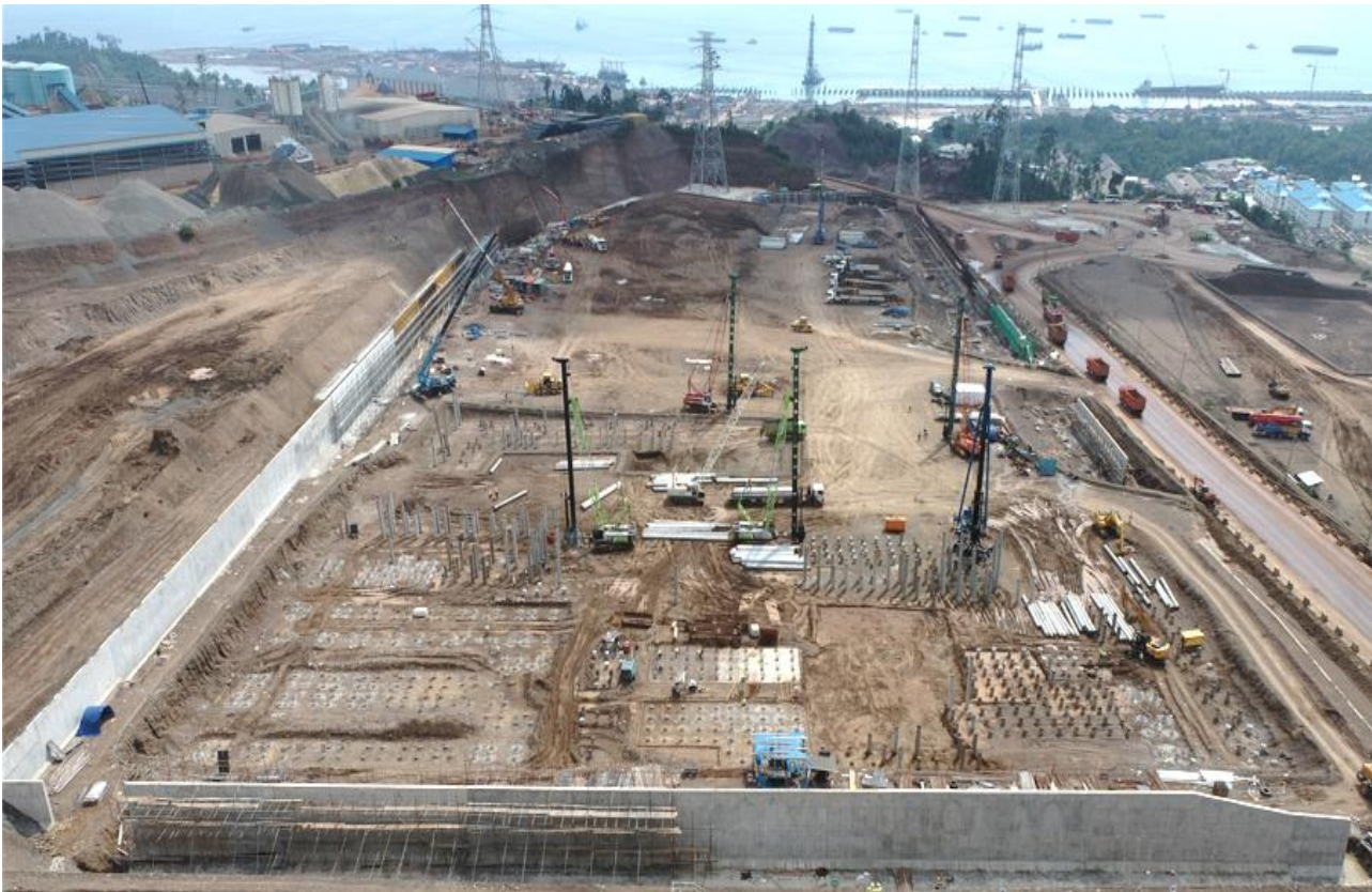
Figure 3: AIM Acid Plant: Perimeter retaining walls, piling for 2 x Acid Trains and Gas Purification
