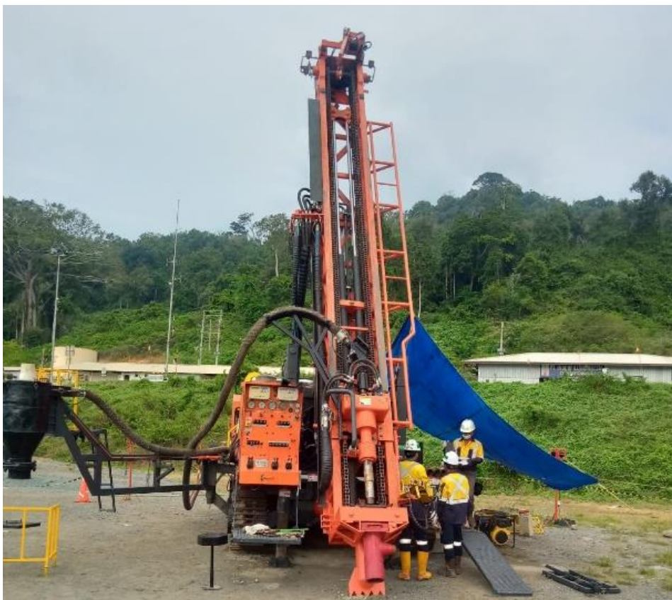
Figure 4: Reverse circulation rig undergoing commissioning prior to commencing drilling at Pit D
